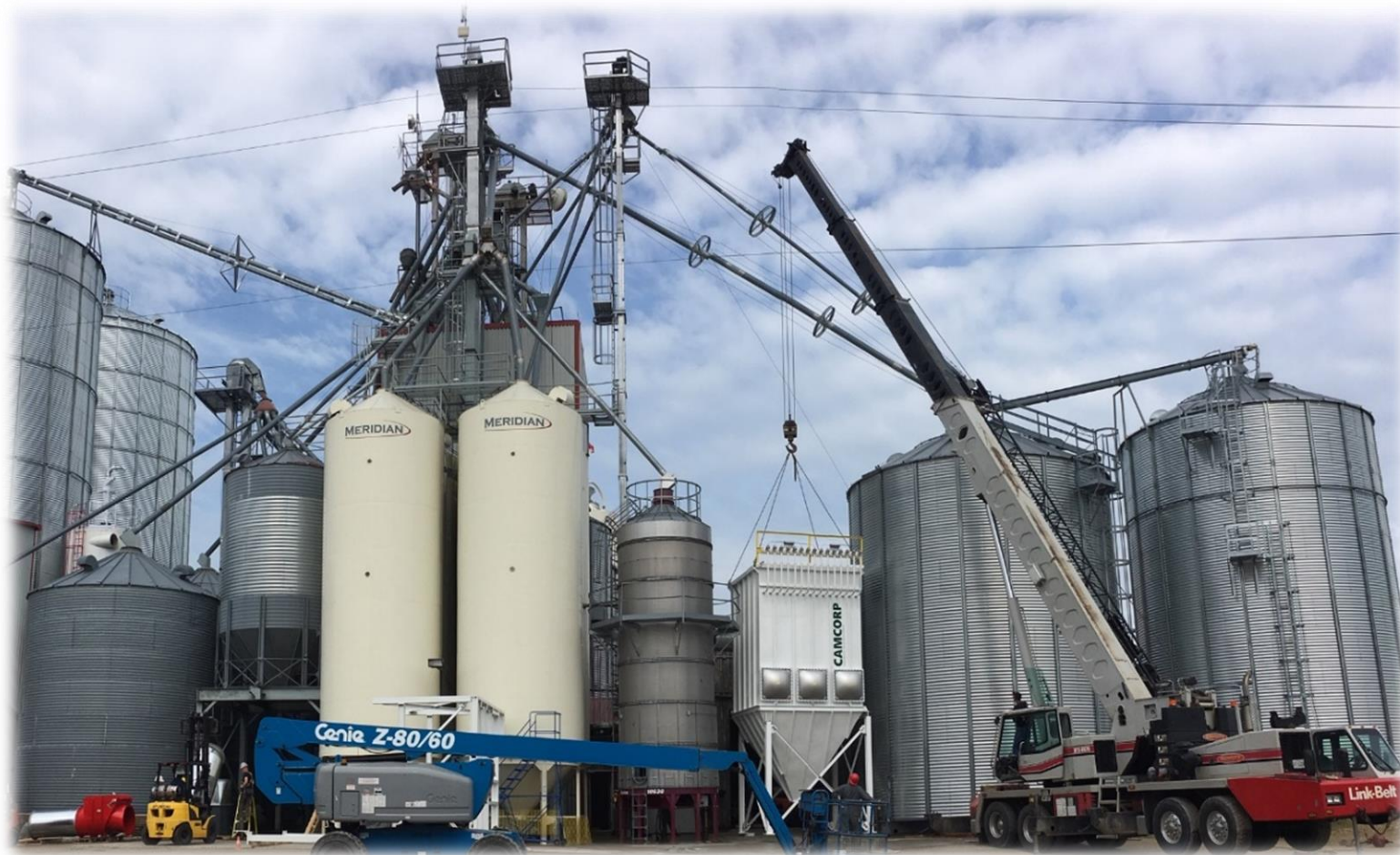
Installation of air quality control system in seed and grain cleaning plant.
